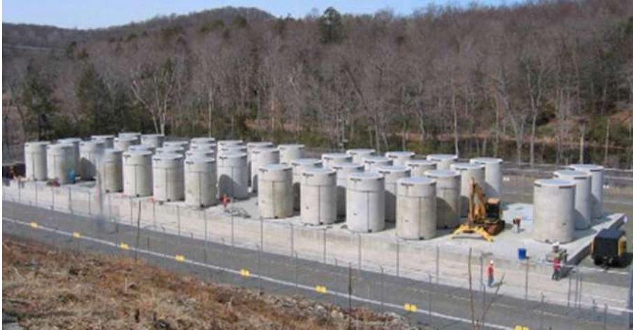
Figure 3.1-1 Concrete casks storing spent fuel at the Connecticut Yankee nuclear power plant site (source: NAC International)
